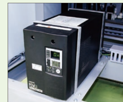
UPS电源 UPS
